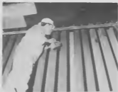
Visual inspection by A. Tromp of HK-40 furnace tubes of H2AR at approximately 30 feet high.
